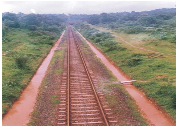
Fig. 116: Pacca drains were provided all along the track in the cutting section for efficient flow of water
